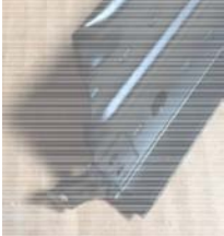
This is bad and should be replaced
