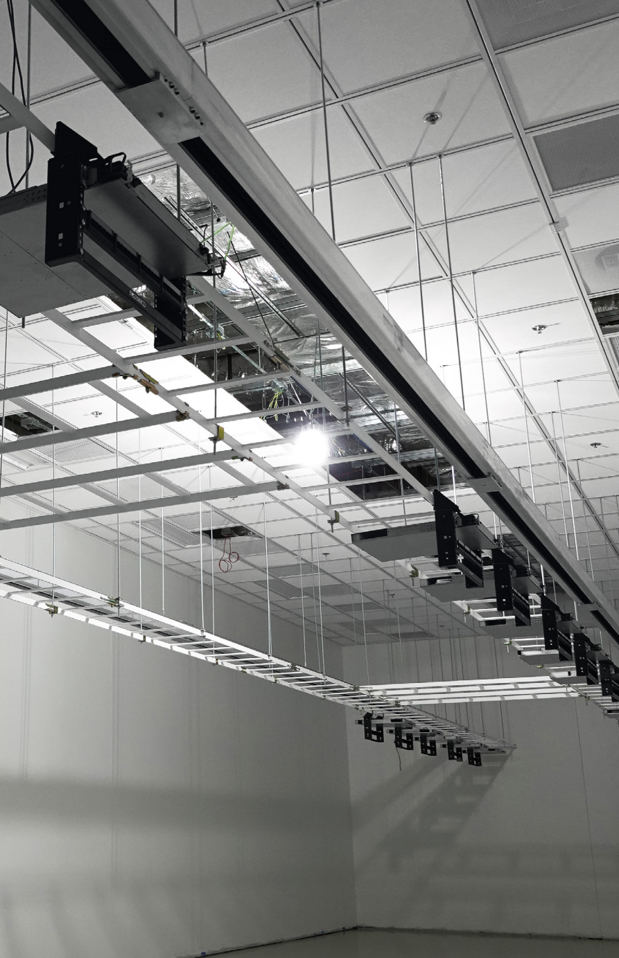
DynaMax® Structural Grid Data Center Installation
