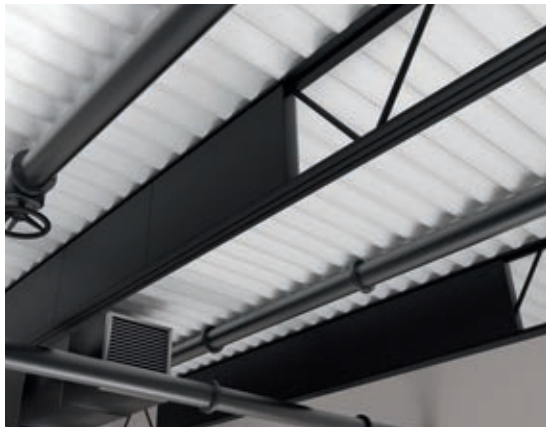
InvisAcoustics™ Panels in Black Truss Installation
