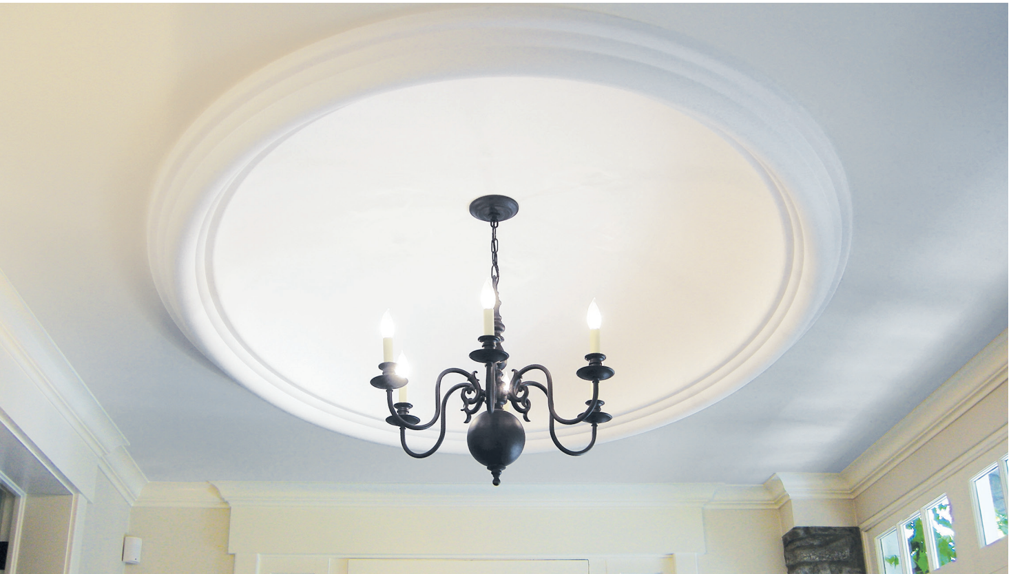
CastWorks GRG interior dome
