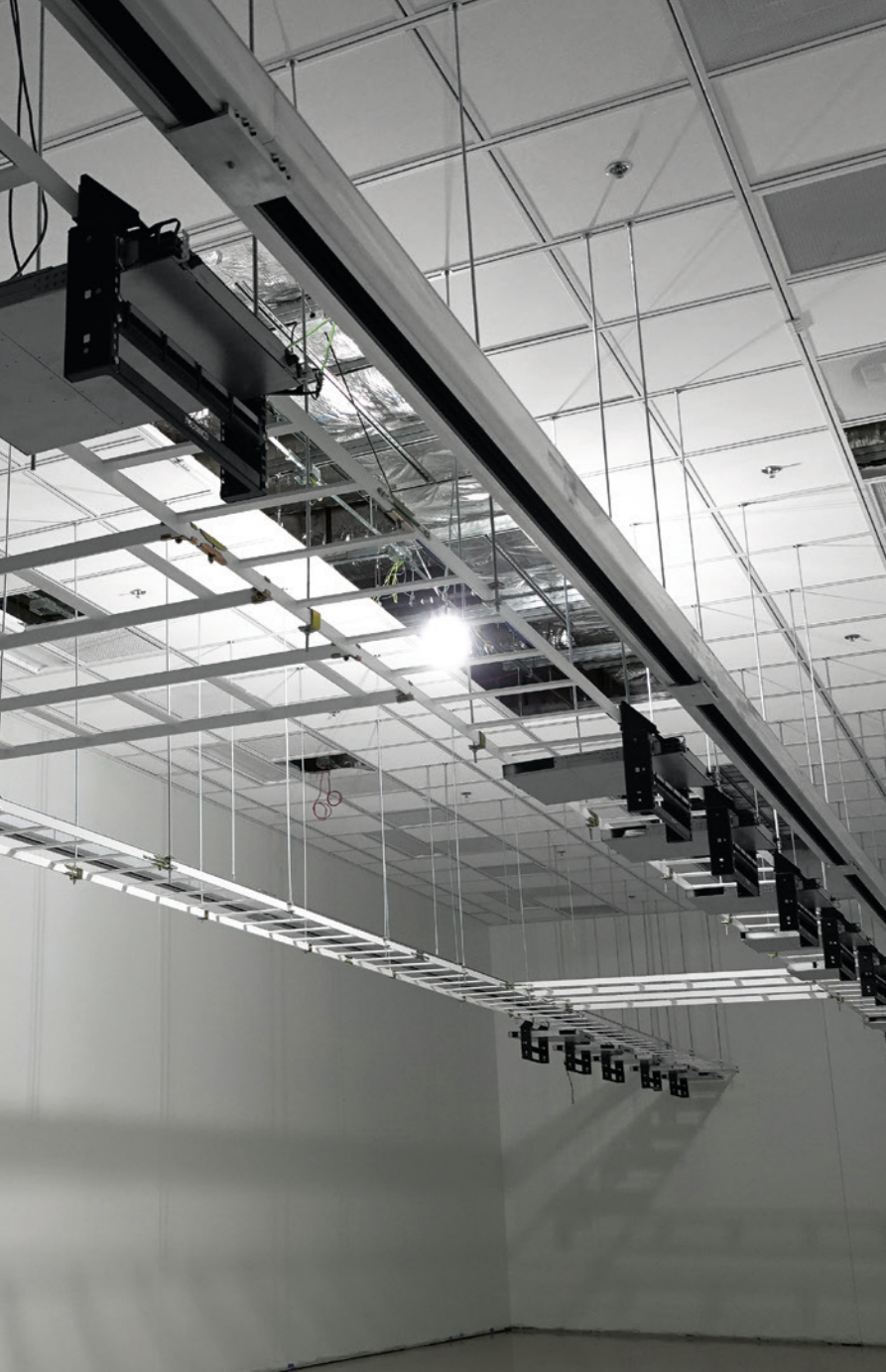
DynaMax® Structural Grid Data Center Installation
