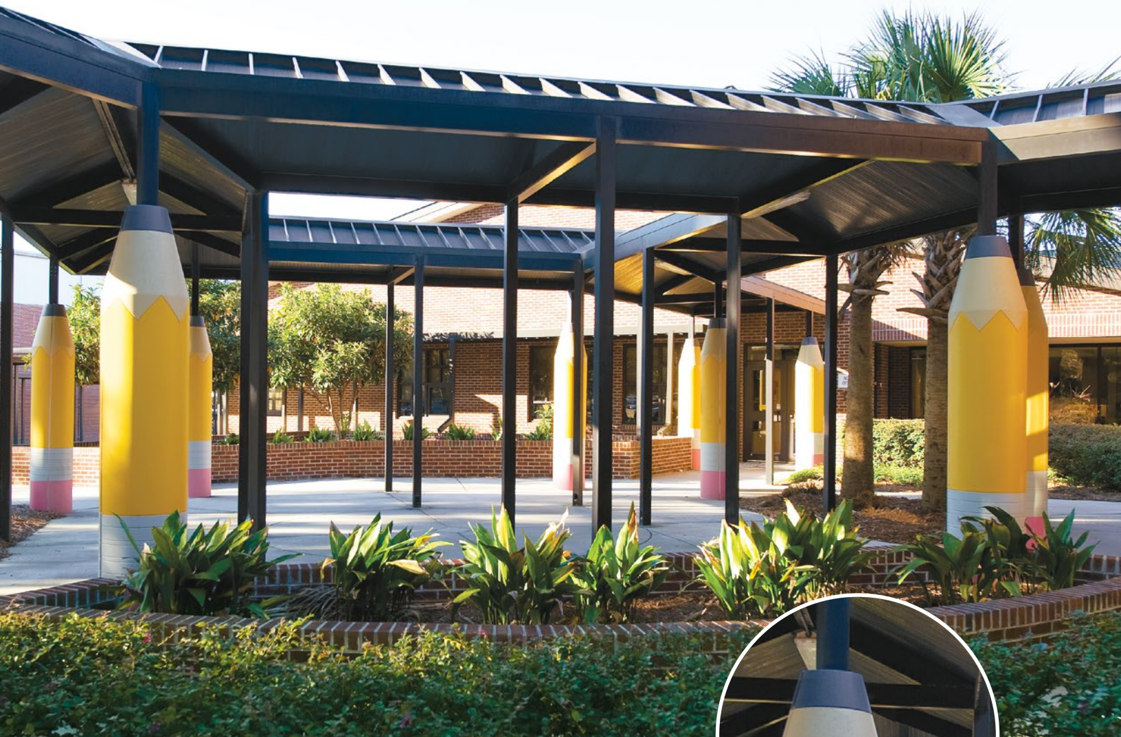
FRP themed column covers; St. Helena Elementary School, Beaufort, SC; Goforth Brown & Associates
