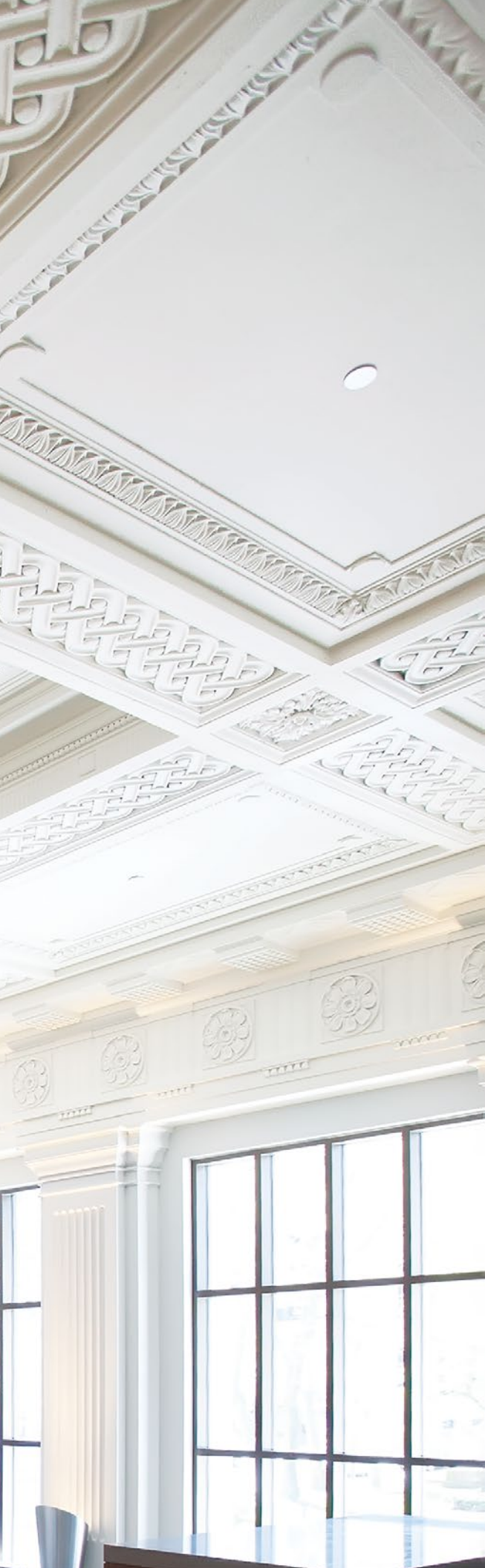
GRG coffers and cornices; The Rockwell Building, Cleveland, OH; Sandvick Architects and Vocon
